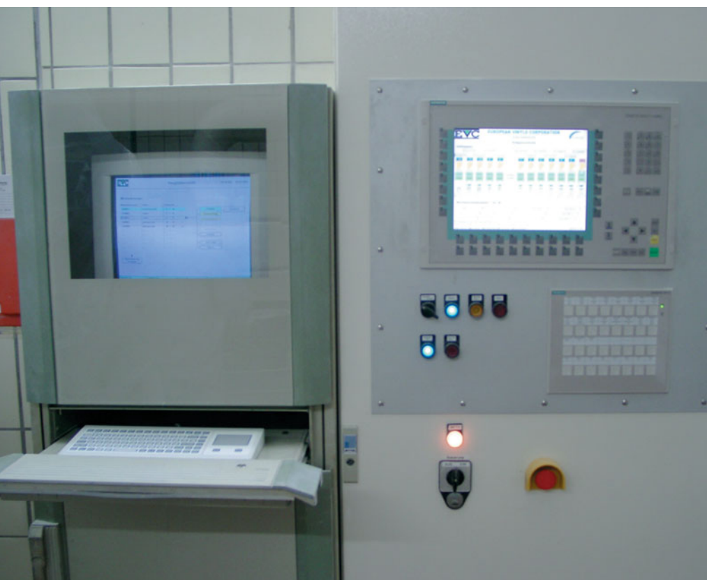
The operator can enter and modify recipes without putting load on the soft PLC executing on the same computer
