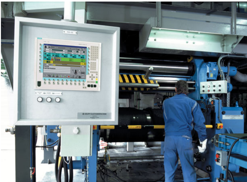
Distributed intelligence: one of three SIMATIC Panel PC 670s at the rolling mill at Krupp Elastomertechnik's development center
